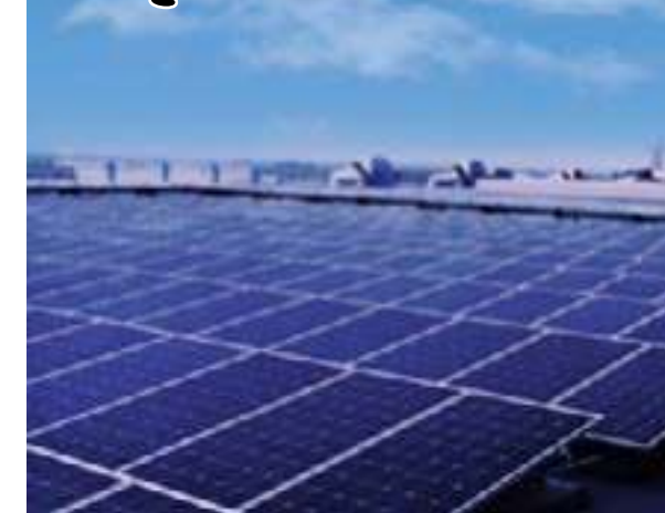
Solar panels are installed across many SM Malls.
