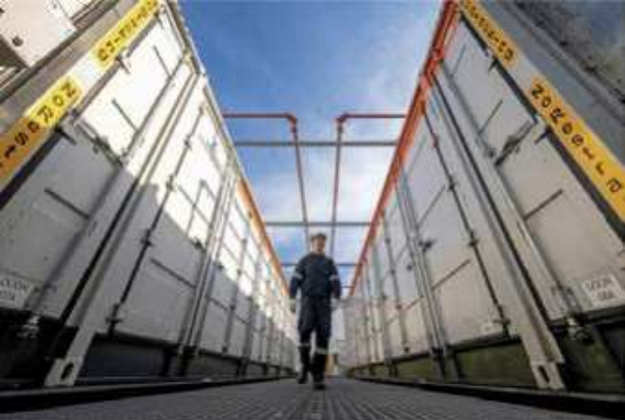
AboitizPower's Battery Energy Storage System supports a cleaner, more sustainable energy future, helping reduce the country's carbon footprint while strengthening power grid resilience—an impactful step in the Aboitiz Group's ESG commitment.
