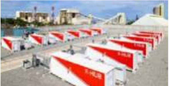
SMC has invested in battery storage facilities throughout the country to help ensure stable, reliable electricity while supporting the integration of more renewable capacities to the grid.
